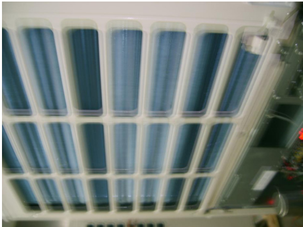
Fig. 10. A photo of no frost on the heat exchanger surface in the nominal heating experiment.
